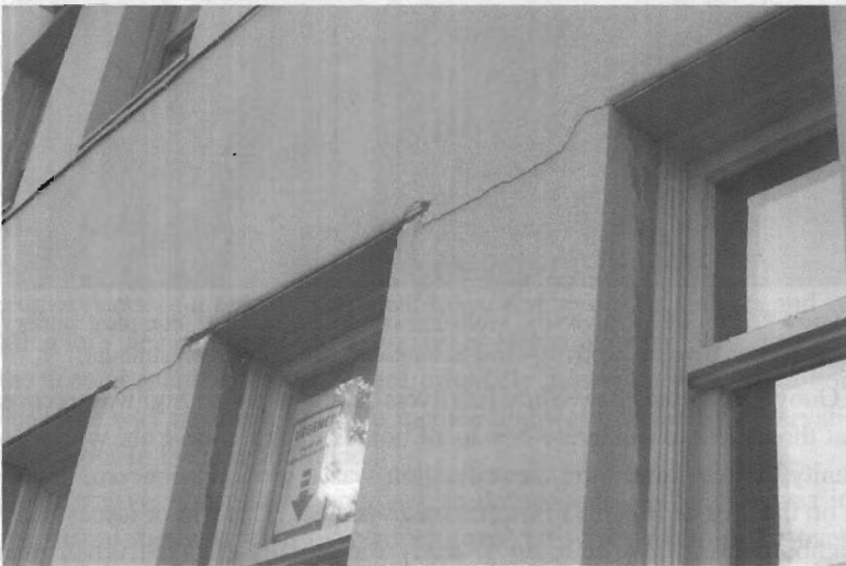
Figure 9.5 Cracks on the façade of highway-adjacent building in Saint-Henri.
